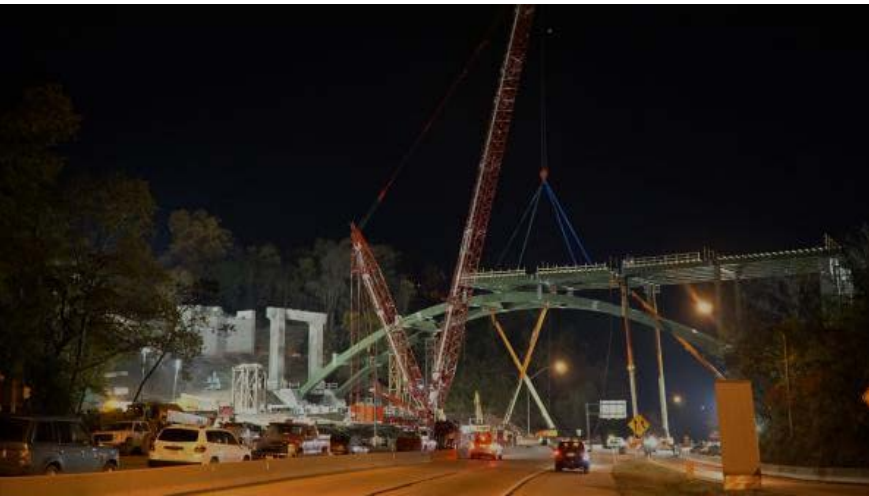
In the photo: Construction is underway on the replacement for the Greenfield Bridge in Pittsburgh. The replacement bridge will open to traffic later in 2017.
